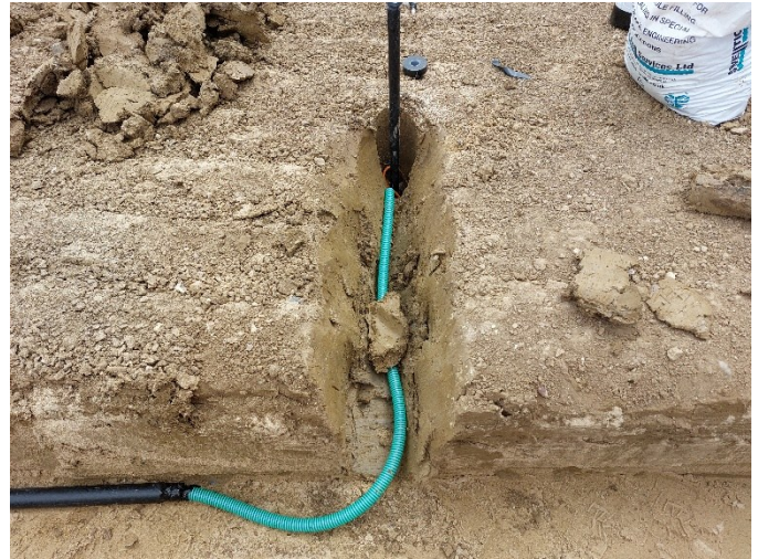
Figure 10: VWP cable protected by flexible conduit and trenched away from borehole towards logger (out of picture to left)
