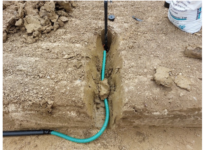
Figure 10: VWP cable protected by flexible conduit and trenched away from borehole towards logger (out of picture to left)
